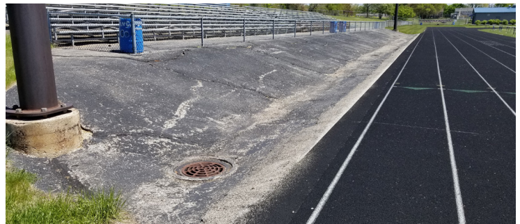
Our track is at the end of its useful life and asphalt and concrete is aged and cracking throughout our district.
