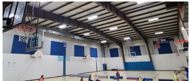
Auxiliary gym in elementary does not have cooling. This causes floors to be slippery and unsafe.
