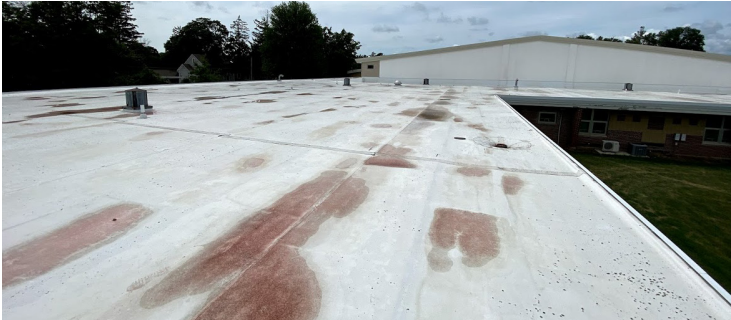
Partial roof replacement is needed at Jr./Sr. high school.
