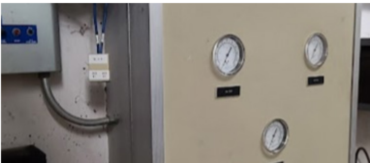
HVAC, mechanical, and controls system is outdated and need to be replaced with an efficient system.
