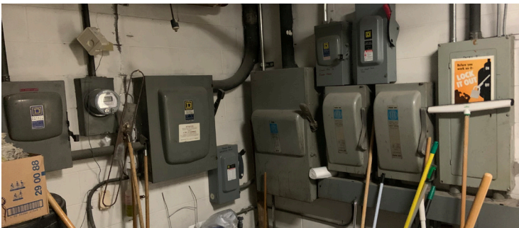
Inefficient electrical panels pose safety and maintenance concerns.
